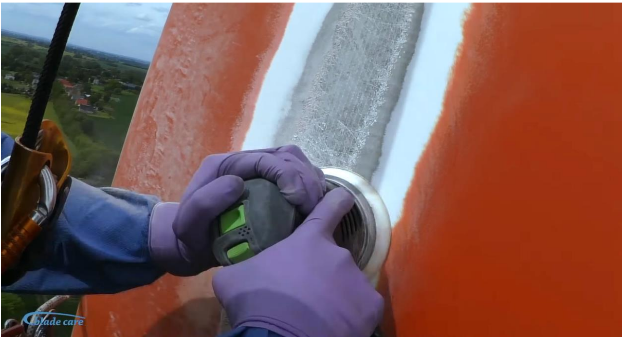
Another example of in-situ repair operation. Same method of open air release of micro plastic and epoxy particles to the environment.
