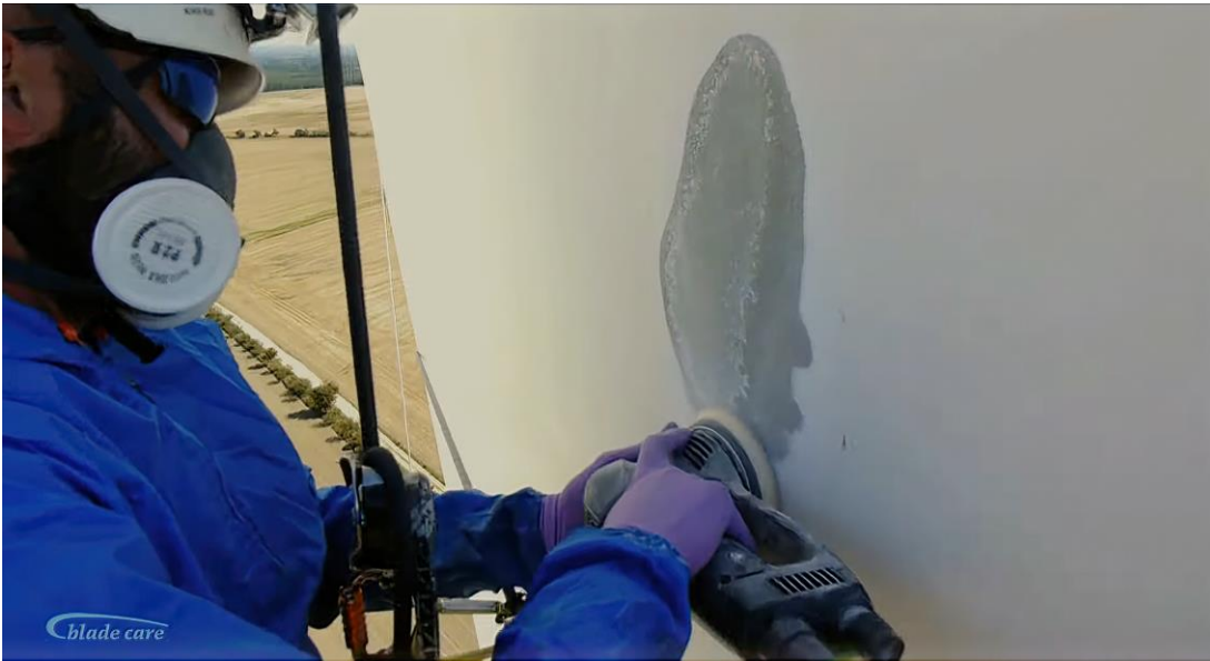
Another example of in-situ repair operation where all particles are released directly into the environment. Please notice the gas mask protecting the operator, while no effort has been established to protect the environment.
